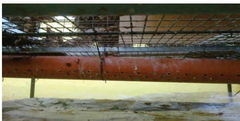
Fig.2. Location of exhaust pipe under the floor of the cage
