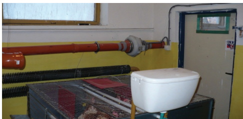
Fig.1. Ventilation technology by conventional method of laying hens.
