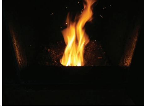
Figure 2. The flame inside the boiler furnace
