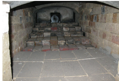
Figure 4. The mobile grate of the boiler
