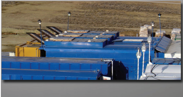
Figure 2. Three E-PODs installed on generators in Wyoming oil and gas fields
