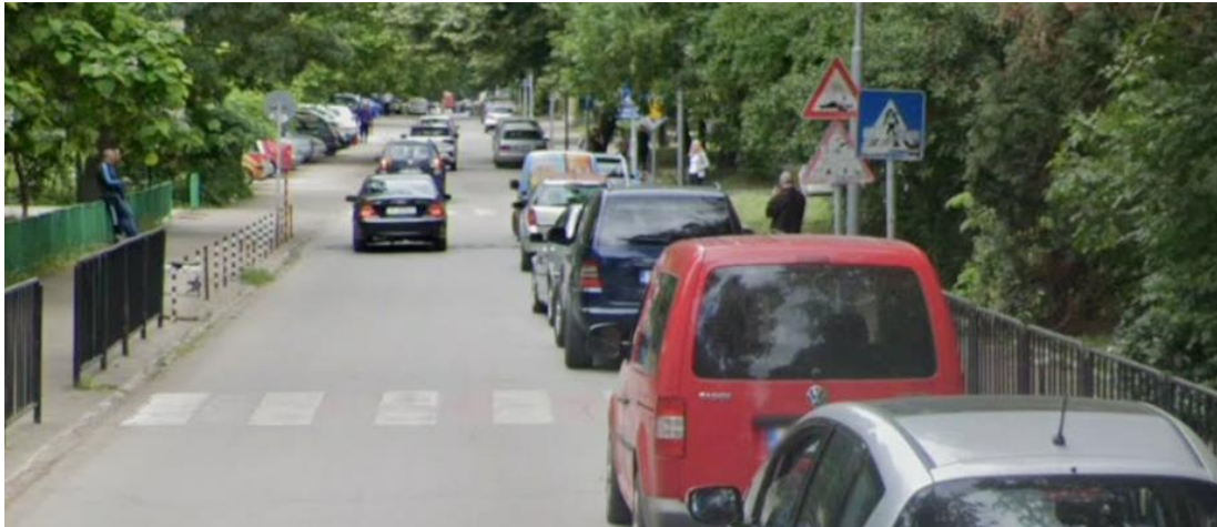
Fig. 2 Pedestrian paths marked only with horizontal markings that are poorly visible and vertical ones in poor condition
